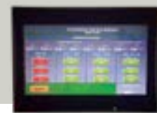
Automated Controls Building Management ANY TEMPERATURE COMMERCIAL - INDUSTRIAL
