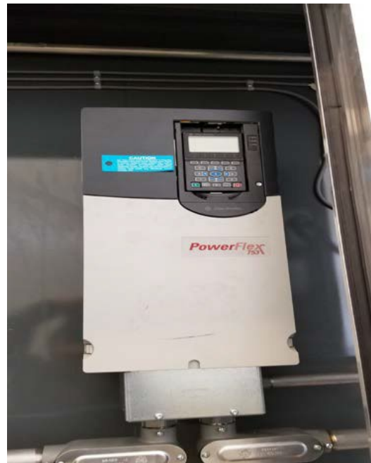
Power Flex VFD
