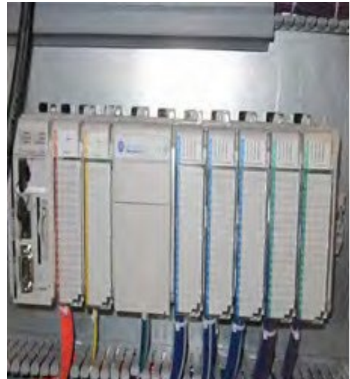
ALLEN BRADLEY PLC
