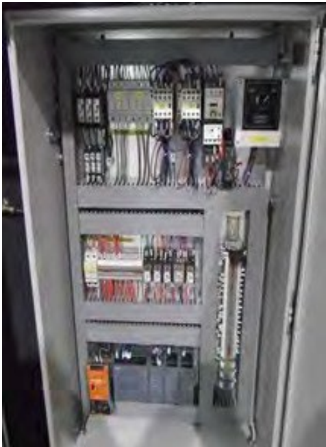
SEIMENS PLC WITH HMI
